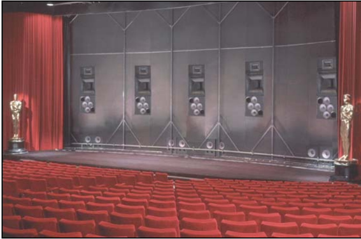
Figur 18: Bakom duken i Academy of Motion Picture Arts and Sciences salong i Beverly Hills. JBL modell 5674, 3-vägs högtalare (deras största).
